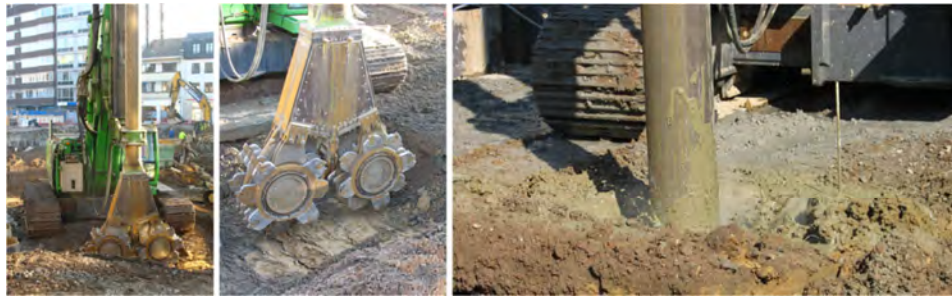
Fig. 2. Execution of a soil mix panel (type CSM) on the construction site of Aalst (Belgium)
