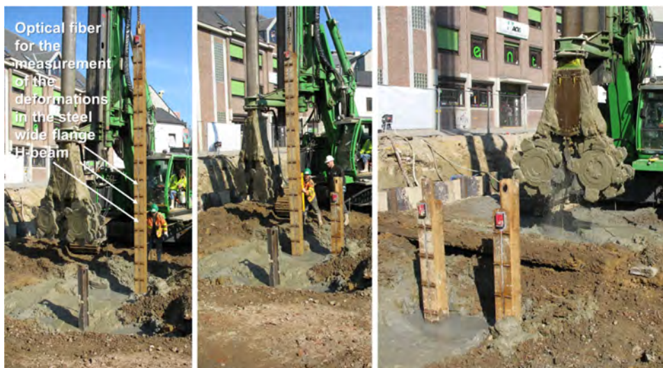
Fig. 3. Installation of the instrumented steel wide flange H-beams in the fresh soil mix panel just after execution on the construction site of Aalst (Belgium)
