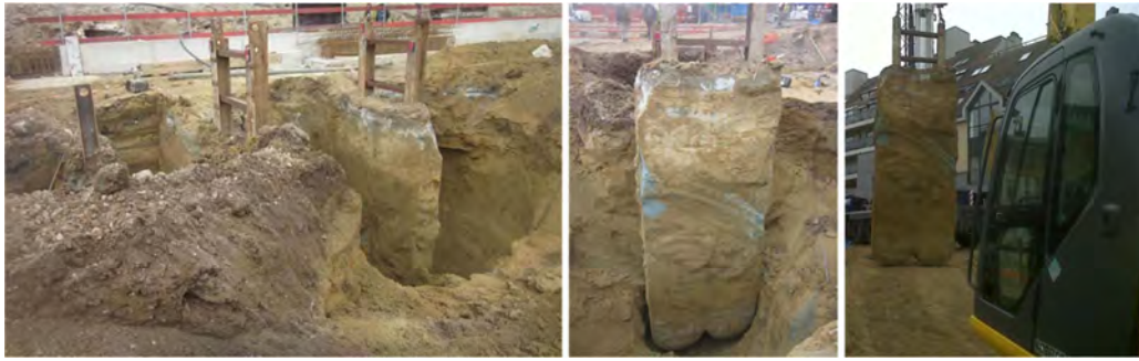
Fig. 4. Excavation of the soil mix panels on the construction site of Aalst (Belgium)
