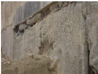
Figure 1: Bentonite/sand-inclusion 1 in diaphragm wall panel
