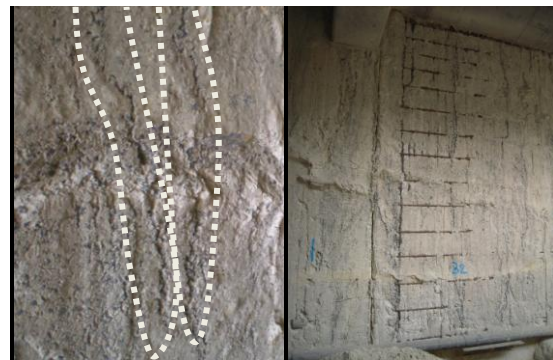
Figure 4: Bleeding channels on the concrete surface and inadequate concrete cover
