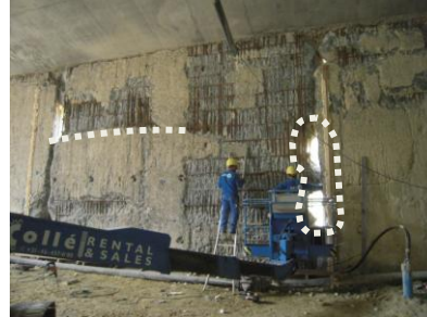
Figure 3: Bentonite/sand-inclusion in joints over the full thickness of the diaphragm wall panel
