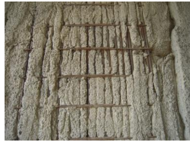
Figure 6: Inclusions caused by the lack of concrete flow
