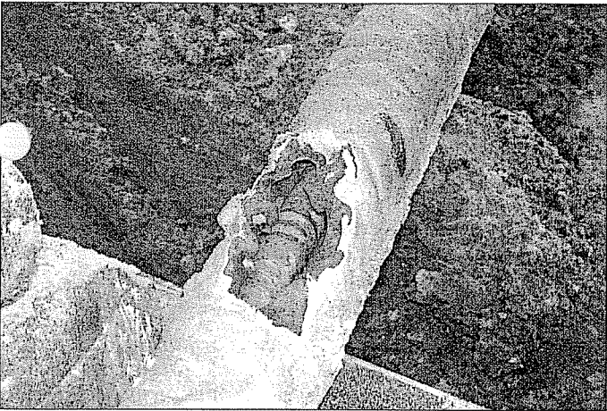
Figuur 8f: Holte in cementomhulling.
