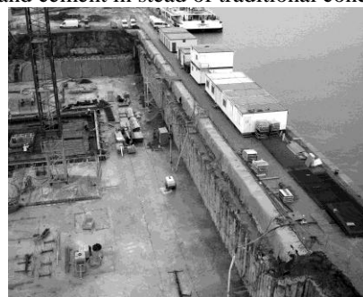
Figure 2. Photo of a soil mix wall with a ground and water retaining function (CVR).
